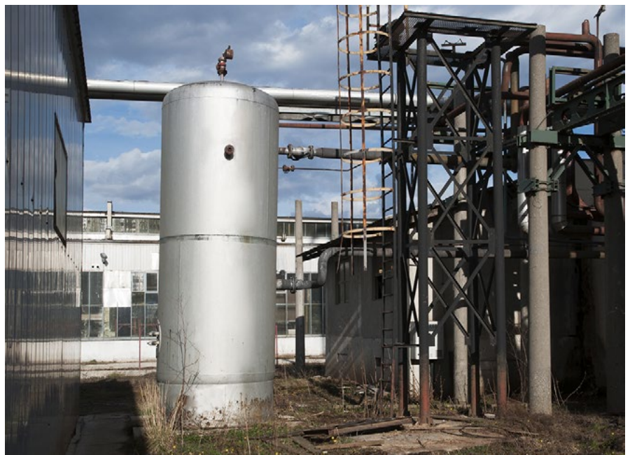
pyrolysis_Gas storage tank2
